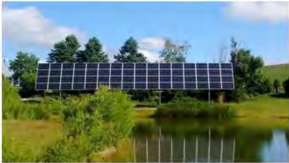
Photo by Master Electrician Jeremy Smith Courtesy of the City of Madison Engineering Division
